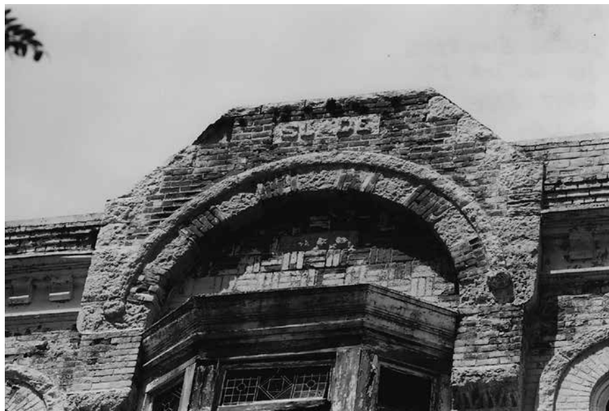
Brickwork on the Slade Block before rehabilitation showed severe mortar damage.
